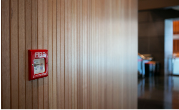
Fire alarms should be installed at locations prescribed in the Building Code.
