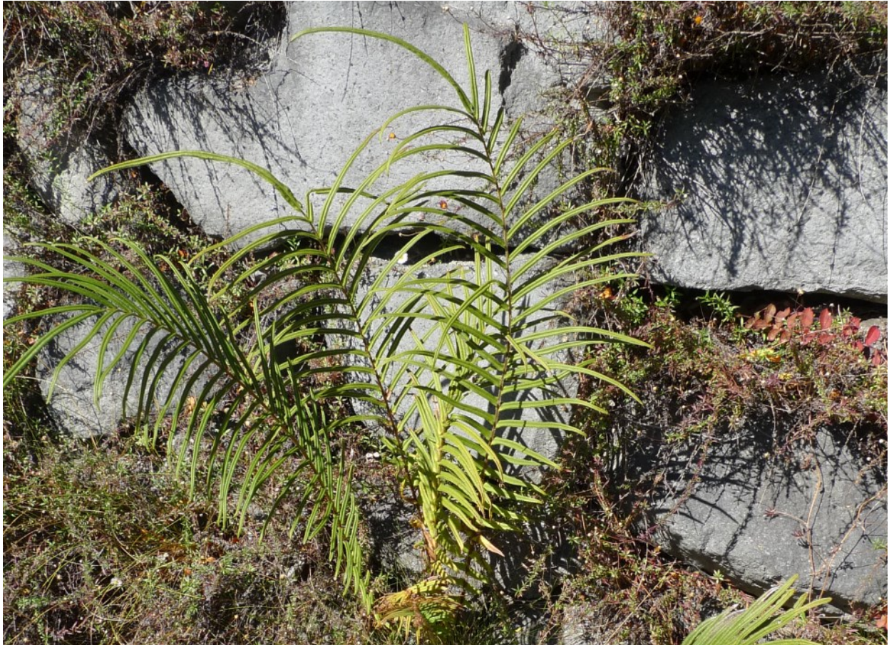
Large plant on retaining wall
